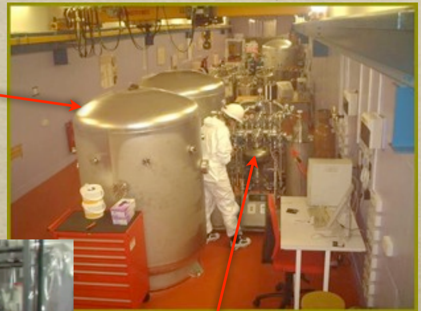
Vacuum, purification and re-circulation systems
